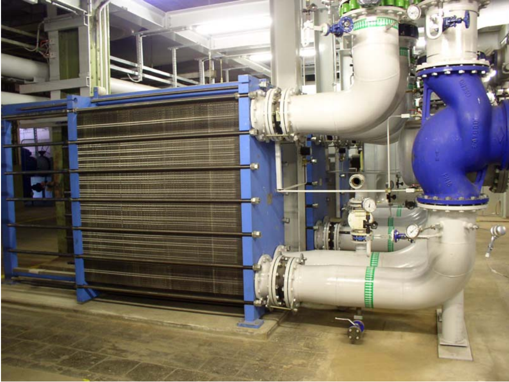
Funke's plate heat exchanger in use by Volkswagen to recover waste heat from their laser welding operation. The waste heat energy is then re-distributed to heat their painting and plant operations.
